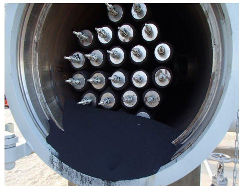
Figure 1. Conventional filter system overloaded with black powder contamination.
