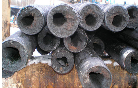
Figure 4. Black powder build up in piping.
