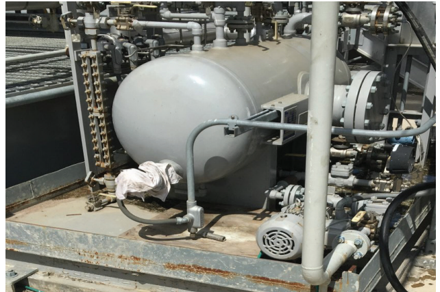
Reclaimed oil tank.
